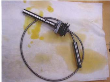
VIEW OF REMOVED OIL QUANTITY MEASURING SENSOR
